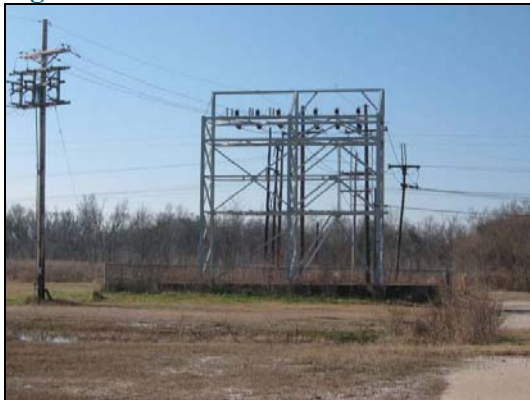
Figure 15: Amax – Electrical Service
